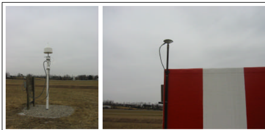
Figure 5-9. Installed High Zenith (left) and PinWheel (right) Antennas
